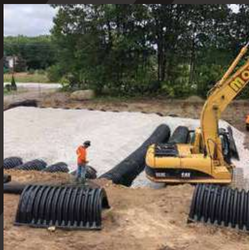
Septic Design & Installation
