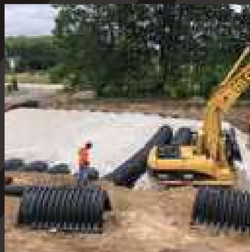
Septic Design & Installation
