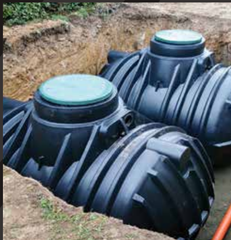
Septic Design & Installation
